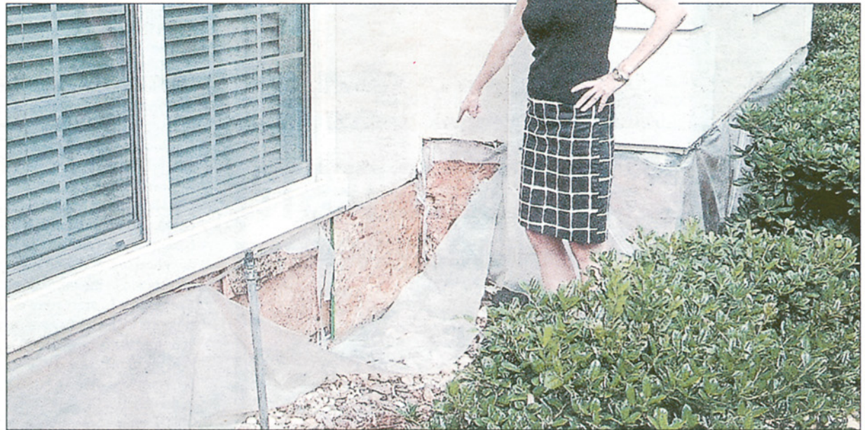
BUGGED: Elizabeth Allen of Ponte Vedra, near Jacksonville, shows the termite damage to her home — after she had hired Orkin to rid her house of the pests
