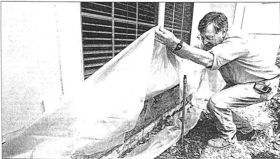
Bob White, a licensed contractor and independent consultant, inspects termite damage outside Elizabeth Allen's home recently in Ponte Vedra. A structural engineer told Allen her house was so damaged by termites that it was prone to collapse if there was a significant storm.
